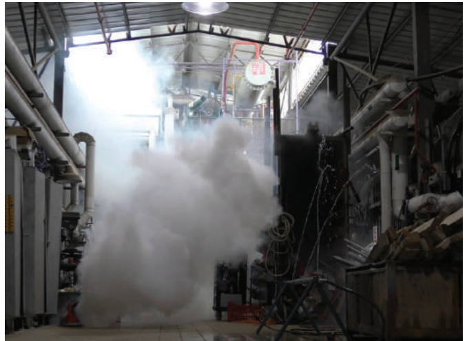
Harmful gas: Ammonia, etc.
